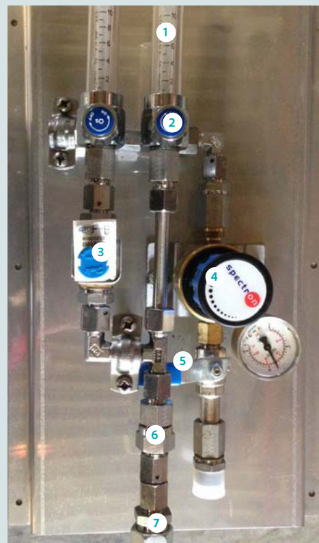
Example of GasDos panel.
